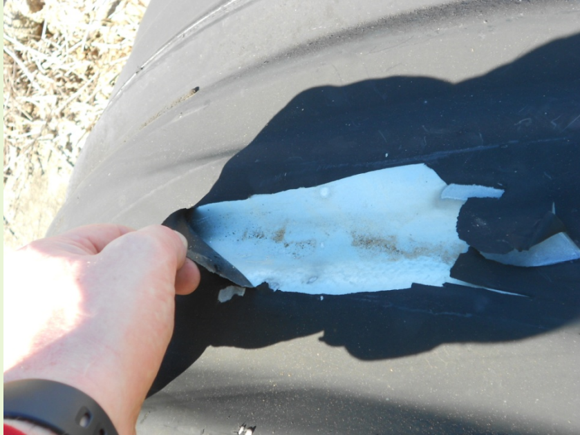
Figure 18. Delamination observed on the exterior of pipe on Joor Rd. likely due to 20 years of UV exposure
