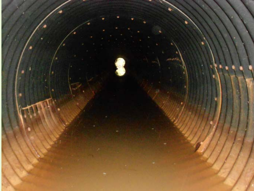
Figure 8. Babcock, WI. Typical good condition of Polymer. The staining on the invert is superficial discoloration from the water line.
