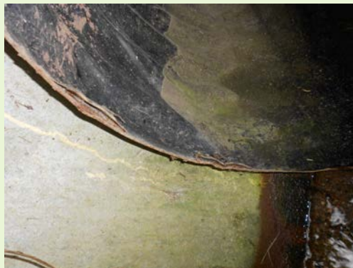
Figure 9. Minor delamination at the outlet of the pipe
