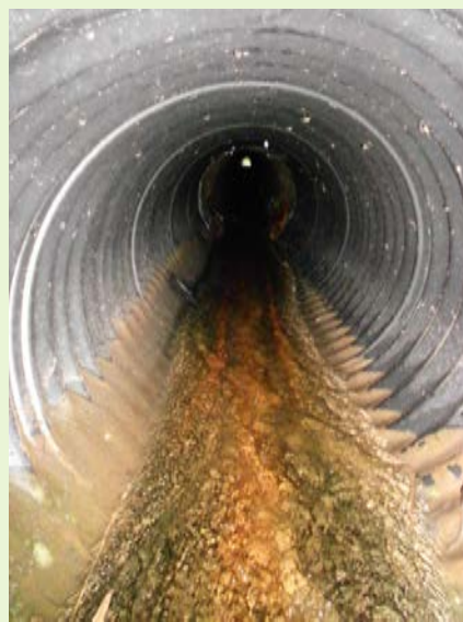
Figure 10. Typical conditions of coated pipe in New York
