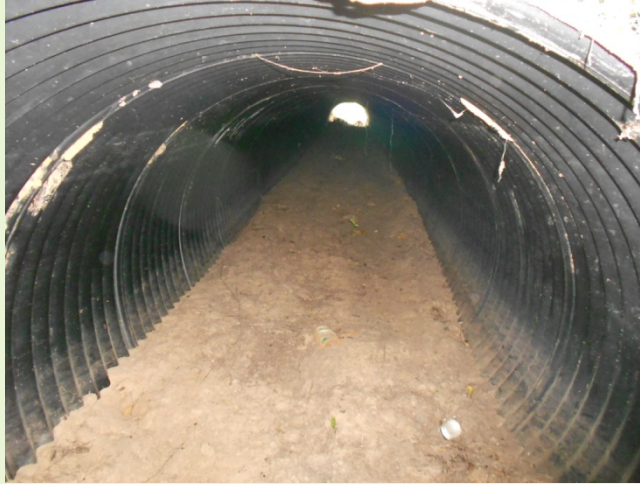
Figure 5. Typical conditions of the pipes in Arkansas
