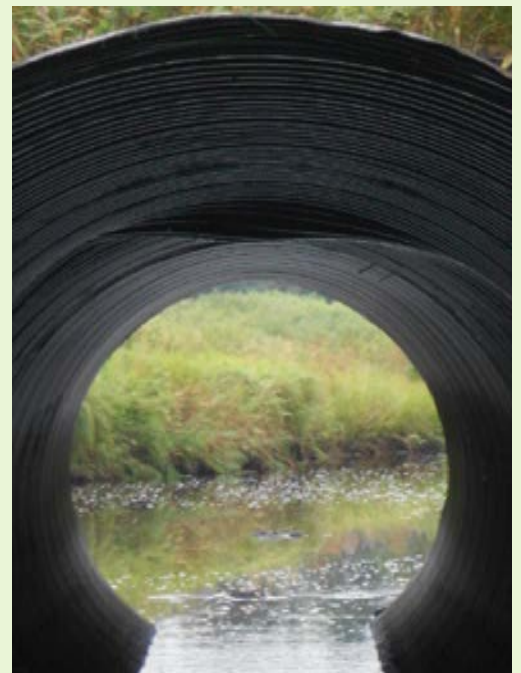
Figure 7. Long Lake installation WI-1. Note the polymer is in good condition. Buckling near the end appeared to have occurred during installation. No associated coating damage was noted.
