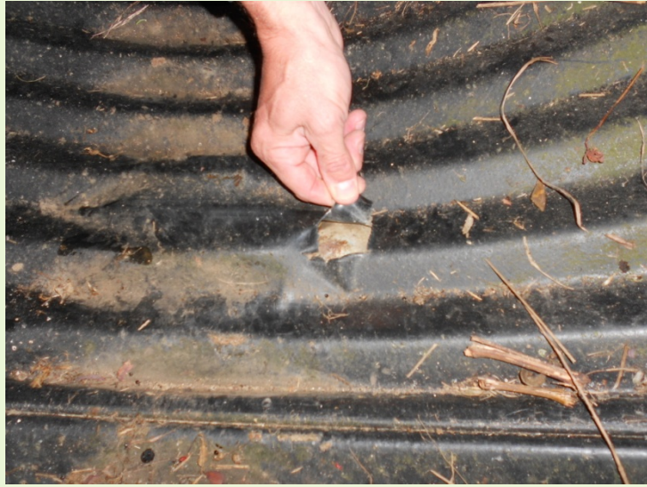
Figure 14. Minor delamination likely due to periodic heavy abrasion and fast flow
