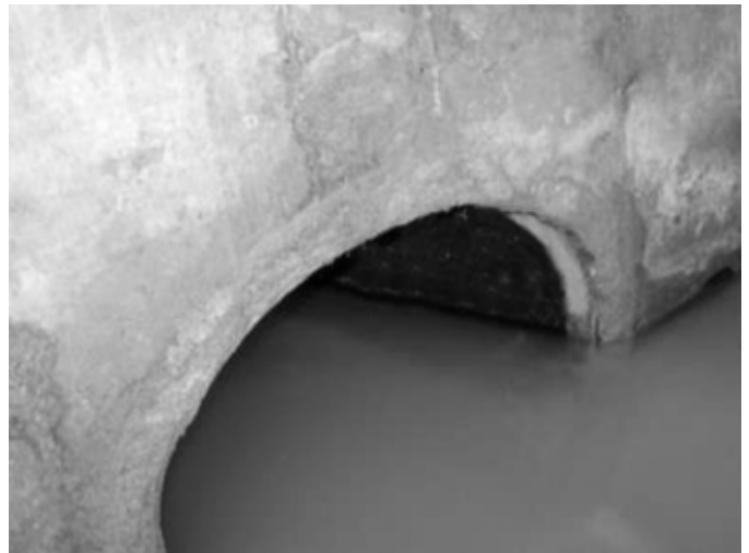
Example of a GOOD pipe installation. Pipe flush with the internal wall of the structure, clean grouting, and proper position.
