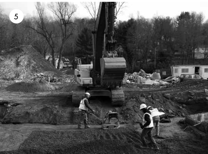
Backfill material is placed and spread from a distance with an excavator.
