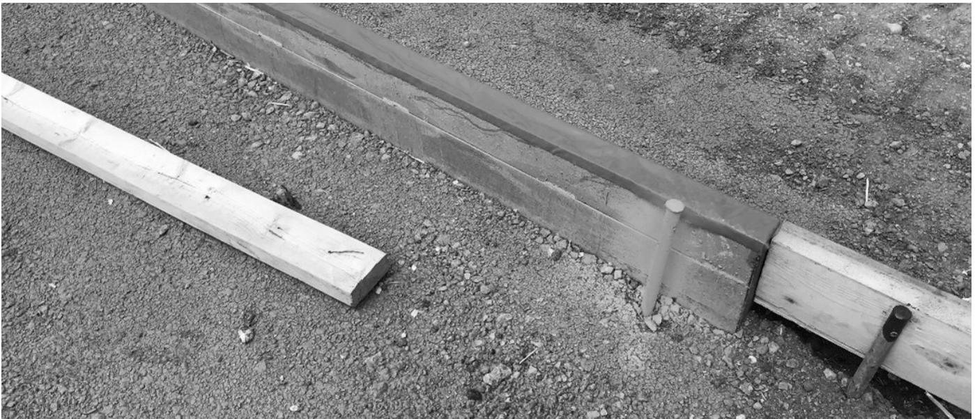
Temporary duct tape can be used to prevent concrete from falling into the grate during backfilling and final paving.
