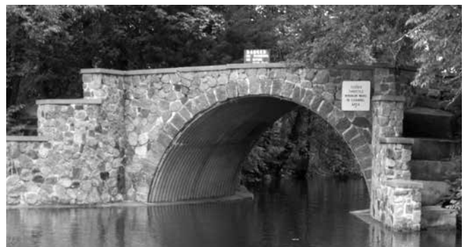
At the time of inspection in 2012, this Steel Structural Plate Single Radius Arch was 72-years-old. Installed c. 1940 | Inspected in 2012
