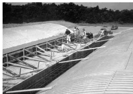
Horizontal reinforcement bars are tied to Contech bent and threaded rods to provide reinforcement for the concrete thrust beam.
