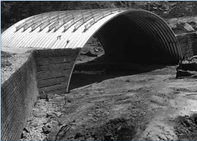
BridgeCor (64'-2" x 19'-7") External Rib System with Vist-A-Wall Welded Wire Wall System during construction
