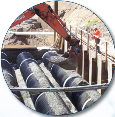
SRPE Tank System
