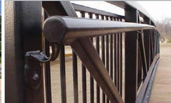
Vertical Picket/Pipe Handrail
